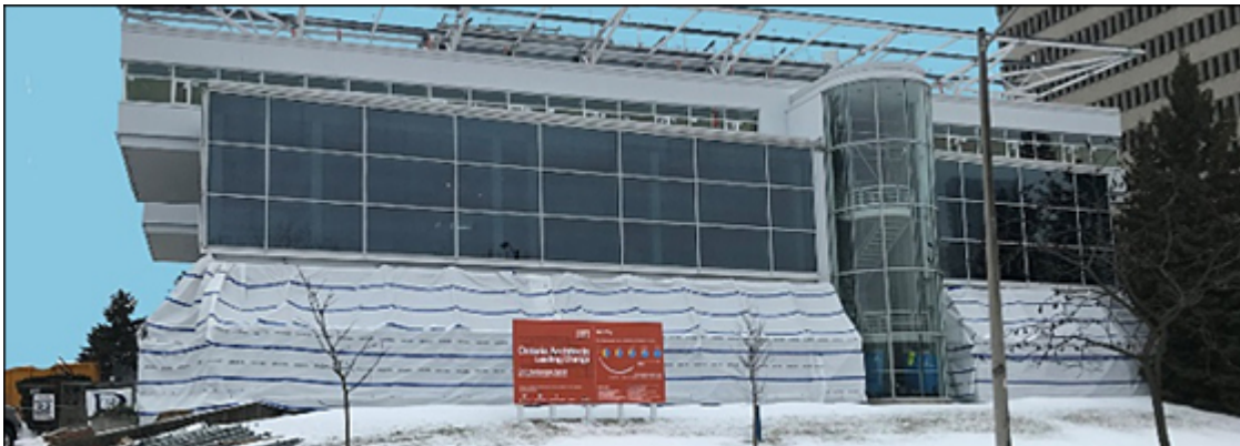
An apron has been installed on the OAA Headquarters, allowing work to proceed on the exterior.
